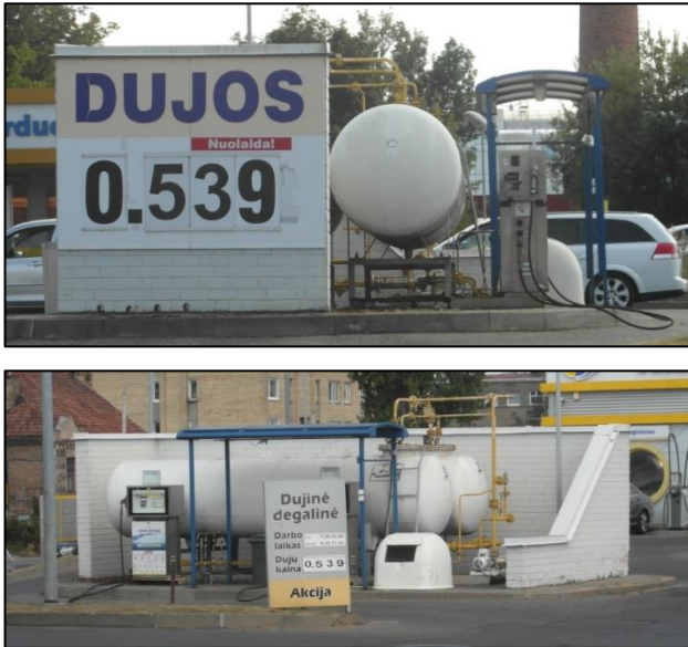
Figure 2. Two photos of a strange masonry structure built as a protective barrier in a petrol station (author's photos)
