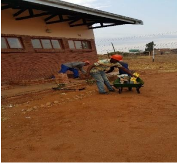
Image 3. After a while, bricklayers had the material to use and all had safety hats
